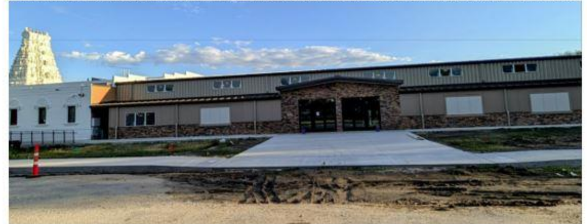
North exterior brickwork; interior wall framing; mechanical, electrical and plumbing rough-in continued
